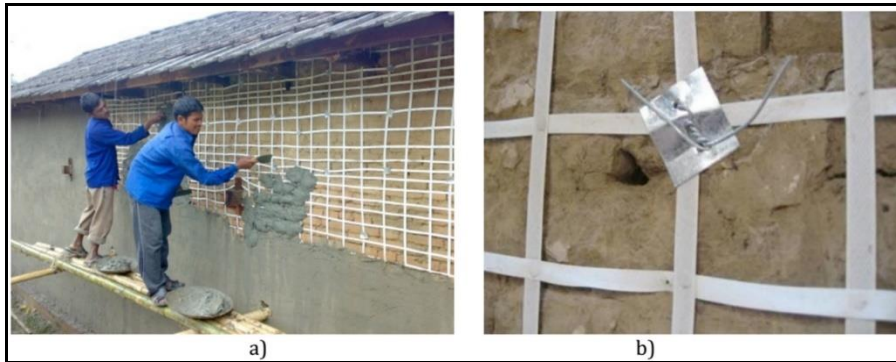
Fig. 4 - a) Implementation of P - P band in Kathmandu Valley; b) anchorage through the wall (Branco et al. , 2014 b).
